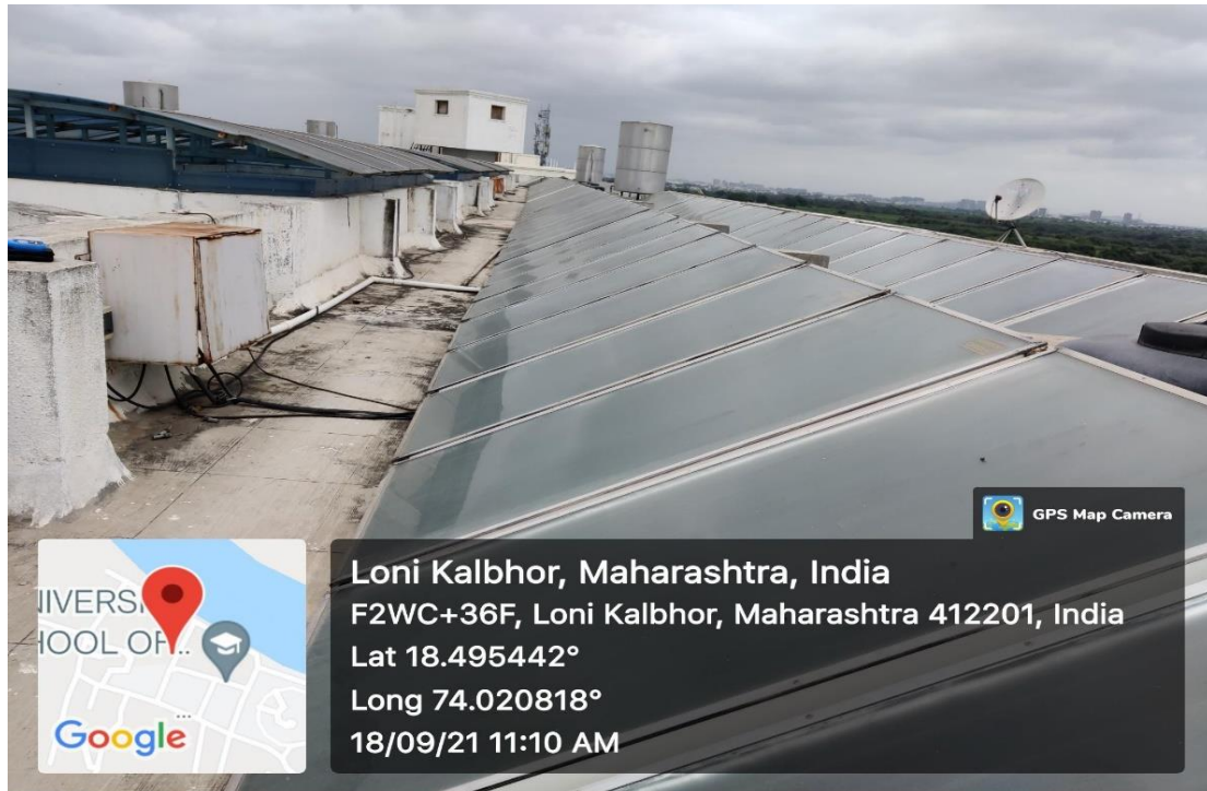
Photograph of Solar Thermal Water Heating System
