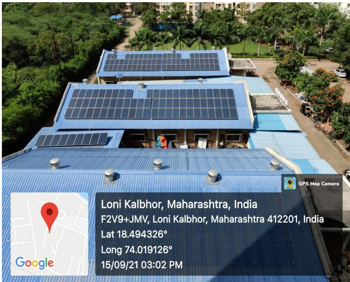
Photograph of Roof Top Solar PV Plant
