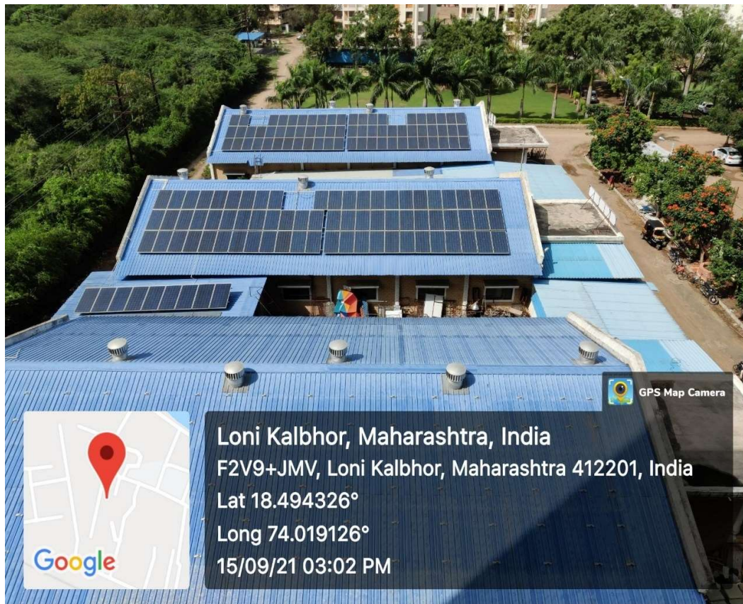
Photograph of Roof Top Solar PV Plant
