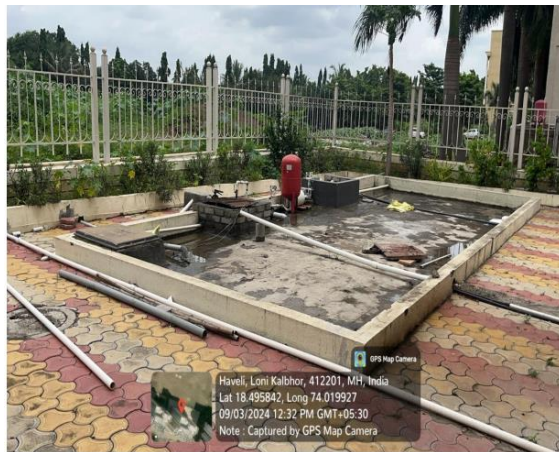
Wastewater Recycle Tank
